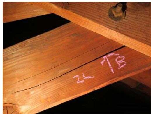
Truss #2 Fracture goes all way through Photo 98
