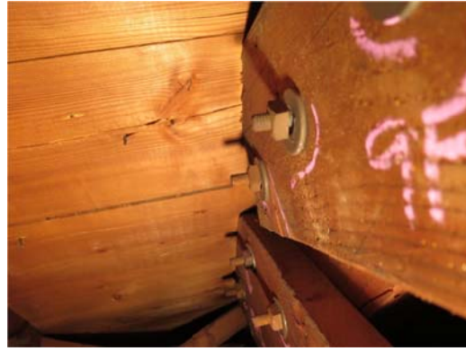
Truss 9 Loose bolted connection Photo 241
