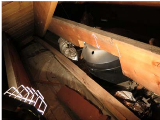
Truss #5 improper notching Photo 176
