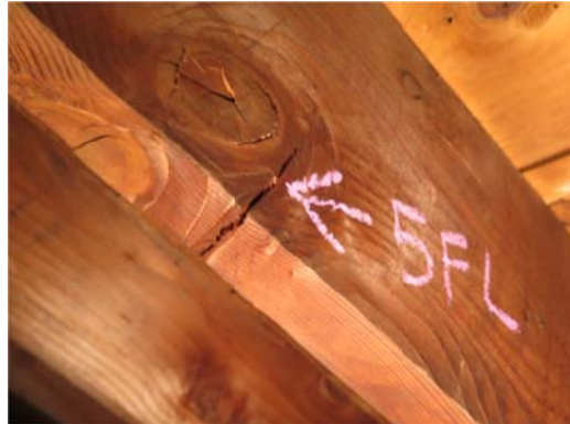
Truss #5 check at knot Photo 182
