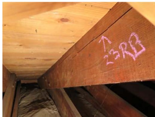
Truss 23 Fractured length Photo 291
