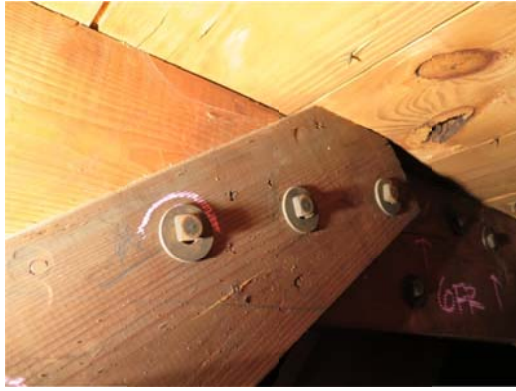
Truss 6 Loose bolted connection Photo 191
