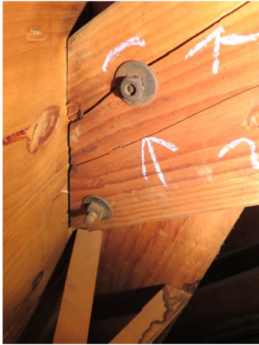
Truss 26 Full fracture through bolt Photo 308
