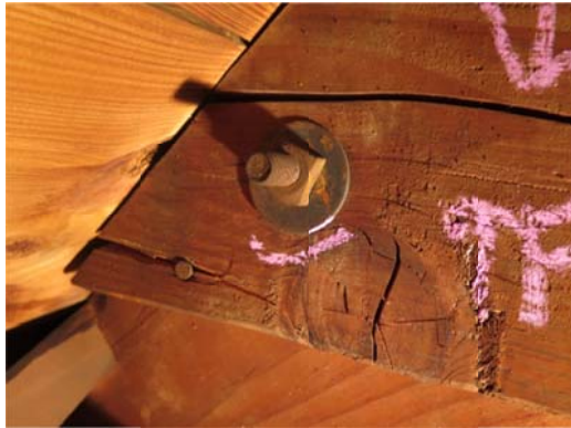
Truss 9 Loose bolt, fractures Photo 243
