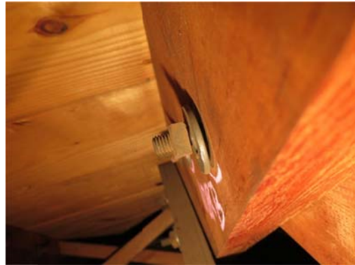
Truss 10 Loose bolt, fractures Photo 215
