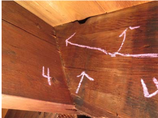
Truss #4 Ridge member split Photo 137
