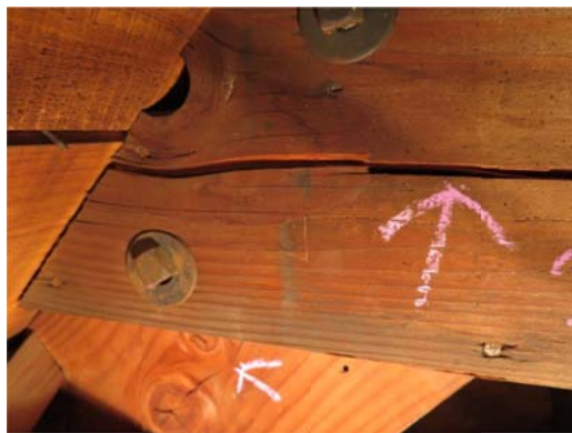
Truss #2 Horizontal member split Photo 130
