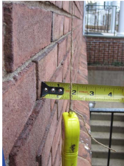
Exterior walls bow out 2"
