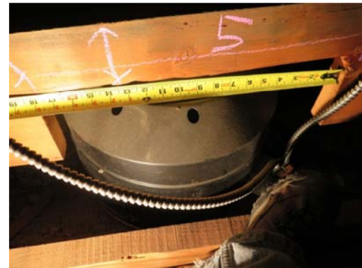
Truss #5 improper notching Photo 175
