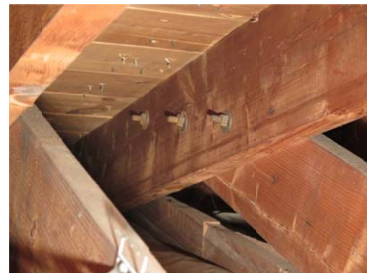
Lowest members mostly intact Photo 161
